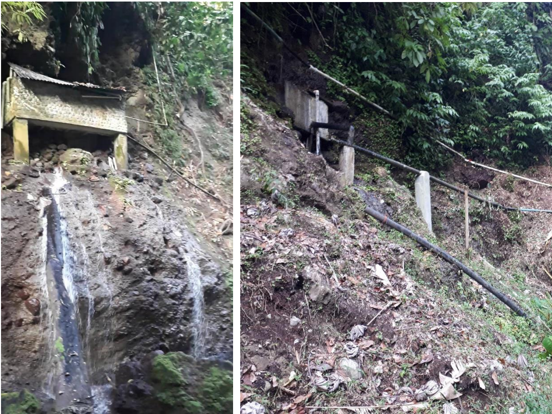
Figure 3.5: Glenelg upper (left) and lower (right) spring collection tanks and gravity feed pipework
