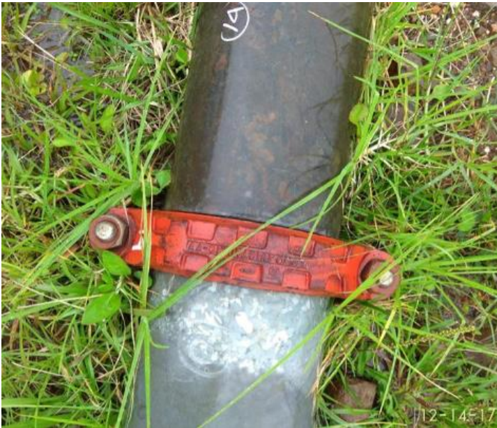
Figure 2.10: Example of temporary carbon steel water pipeline with connection clamp in geothermal drilling
