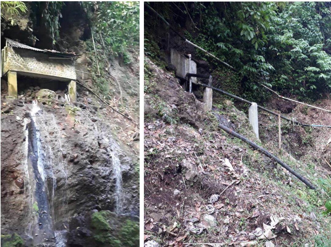
Figure 9.17: Glenelg upper (left) and lower (right) spring collection tanks and gravity feed pipework
