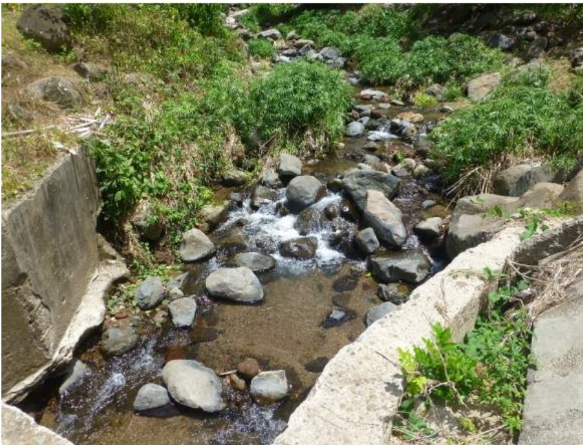
Figure 9.5: Mt Reuil Stream looking upstream from culvert adjacent to the Glenelg bottling plant.
