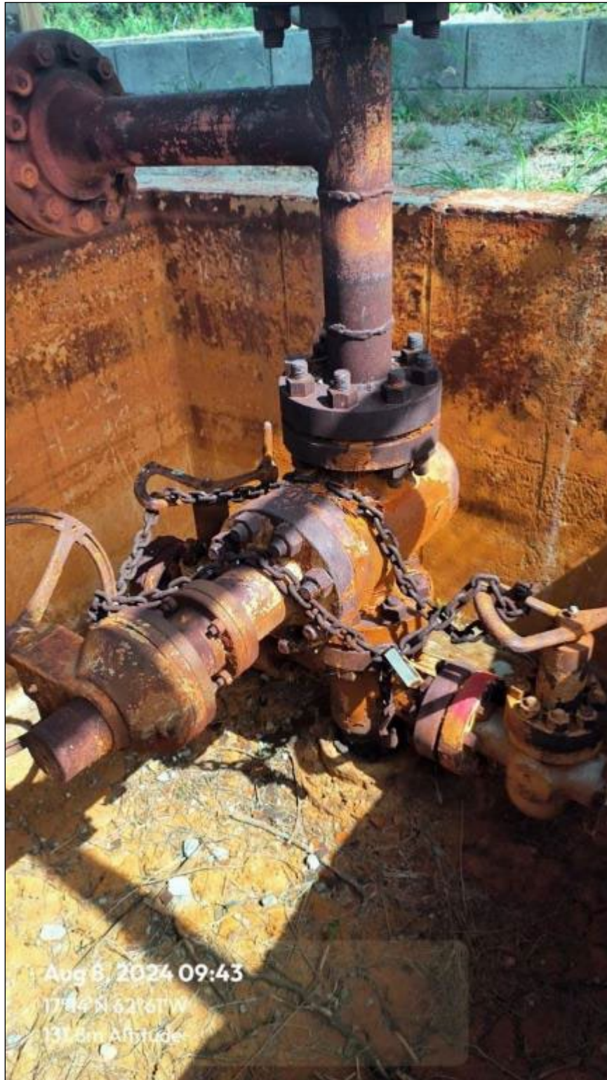
Photo 6: Well N-4 and cellar.
