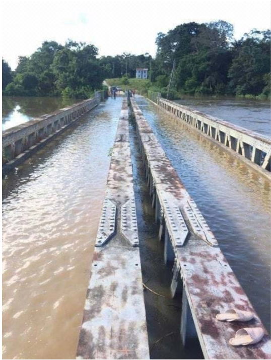
Rancho Dolores Bridge impassable
