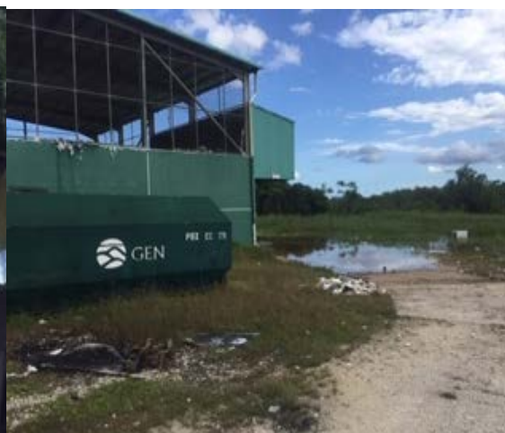
Fig 11: Transfer station inundated
