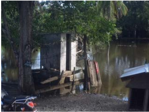
Pit latrine inundated
