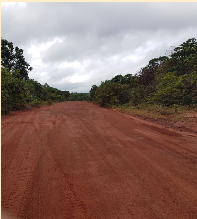
A section of road between Linden to Mabura Hill, which will be upgraded, using SDF resources
