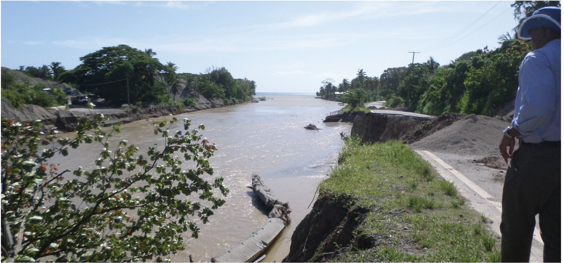
CDB staff examining the damage caused by Tropical Storm Erika to the Layou West Road.
