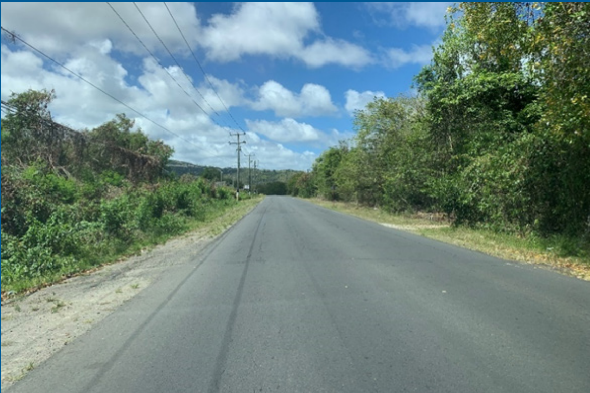
Figure 64: Section of Micoud Highway Without Road Markings
