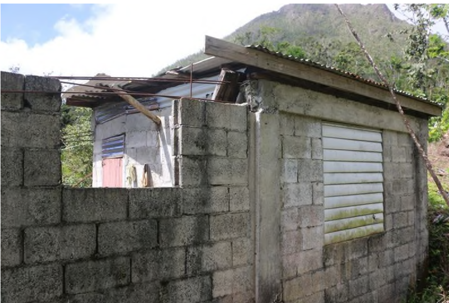
Figure B.4 : Residential Structure Incomplete C3
