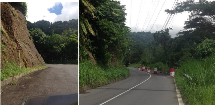
Figure 3.29 : Road signage on Valley Road (left) and image showing a section of the road which is collapsed (right) (Source: Jacobs, 2016).
