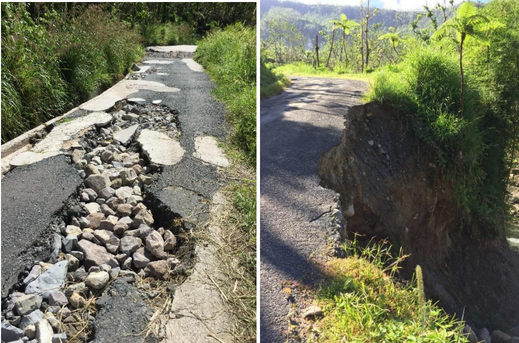
Figure 3.40 : Landslip on the road (right)
