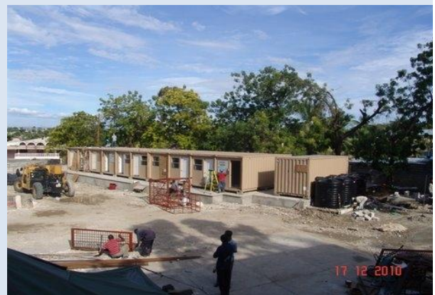
New Temporary Offices under construction for GOH agencies within the Ministry of Public Works, Transport and Communications
