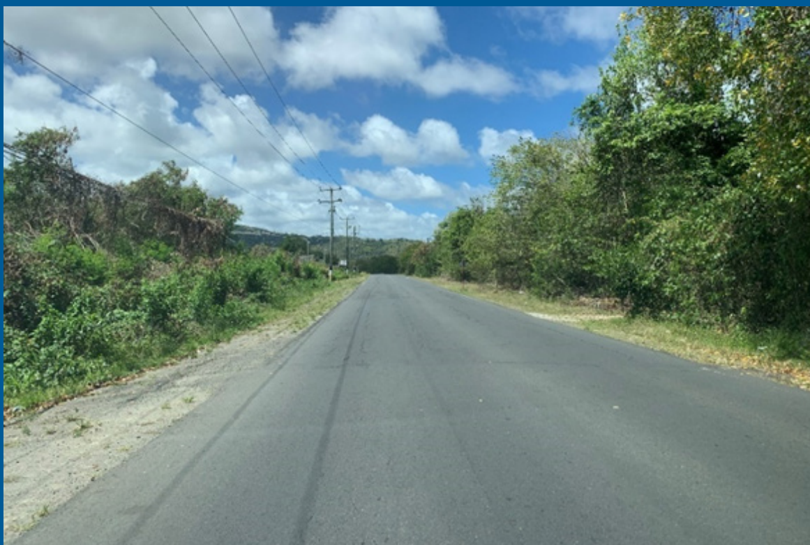
Figure 64: Section of Micoud Highway Without Road Markings
