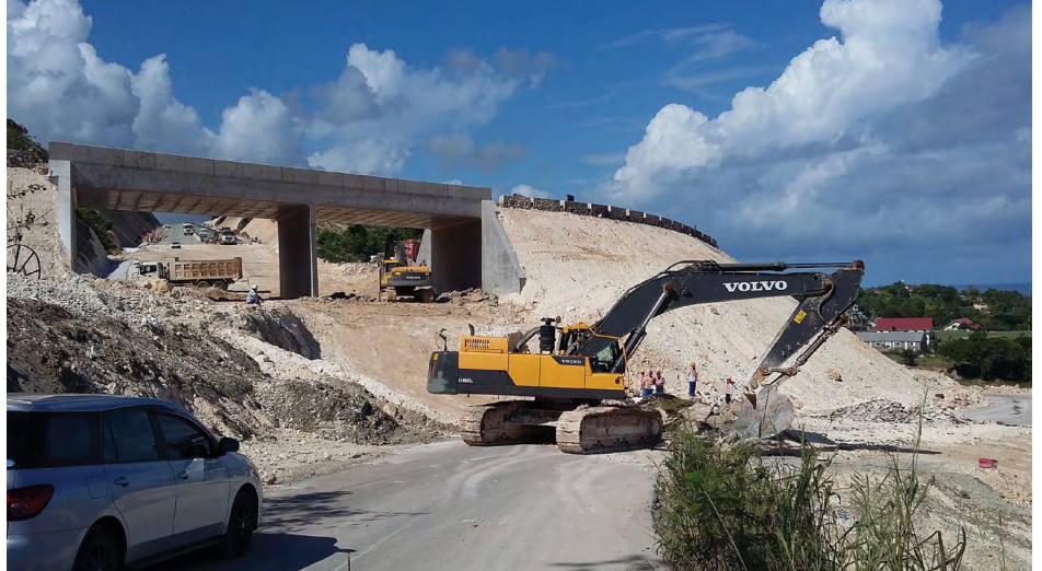
Construction work on the North-South Link of Jamaica's Highway 2000 Project, from Spanish Town to Ocho Rios. The second phase of the Project is a 50-year Concession, held by China Harbour Engineering Company (CHEC).
