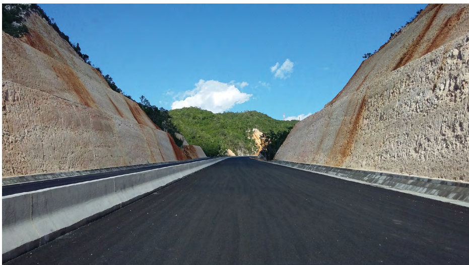
The North-South Link of Highway 2000: a PPP that overcame major technical challenges in Jamaica’s mountainous interior.
