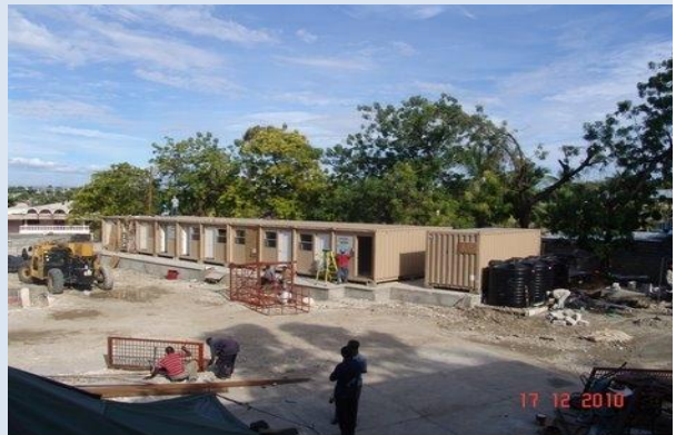
New Temporary Offices under construction for GOH agencies within the Ministry of Public Works, Transport and Communications
